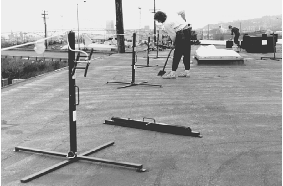
FIGURE 3-7 Warning line system.
