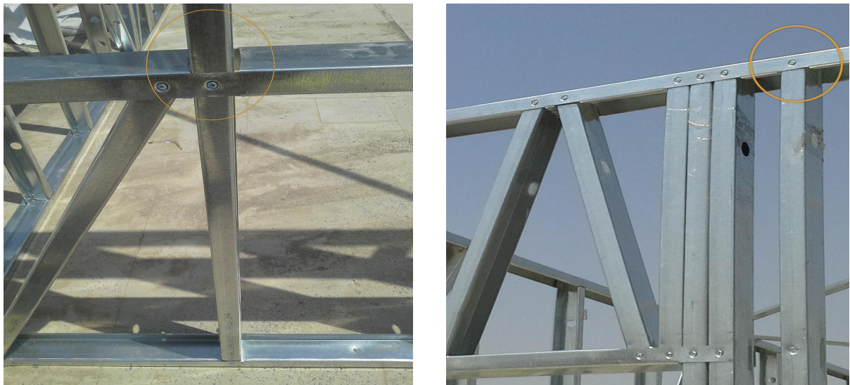
Figure 5: The Connection of Bridge to Stud (Left) and The Connection of Stud to upper Track (Right)
